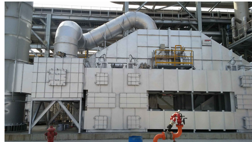
Yantai Campus uses a regenerative thermal oxidizer (RTO) to oxidize and decompose volatile organic compounds (VOCs) in exhaust gas.
